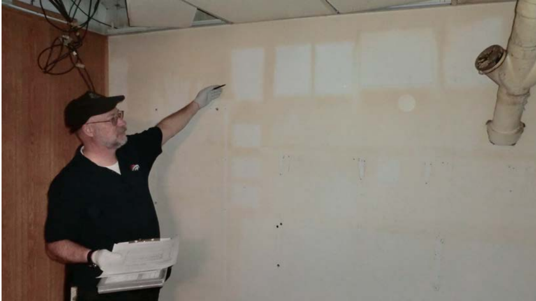
FACTs Photograph - S. Lincoln St., Denver, CO Iodine Staining Basement Living Room
